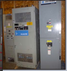
ALLEN BRADLEY MAIN PANEL
