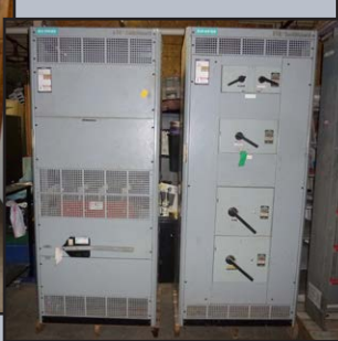
SIEMENS 1600AMP SWITCHBOARD
