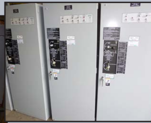
(3) ASCO TRANSFER SWITCHES
